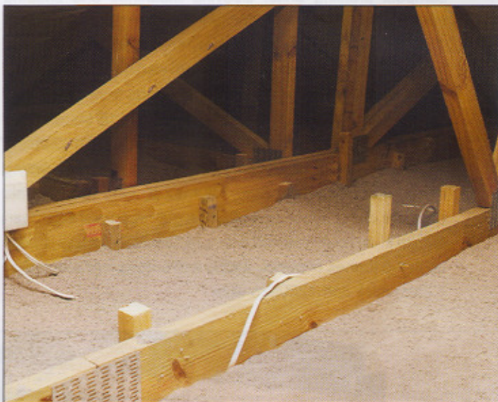
PHOTO by Gareth Griffiths – shows the user friendly product in place in the ceiling, where it quickly mats together and stays there
